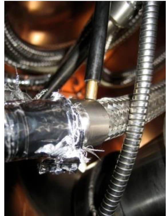
Faulty cooling circuit Located in distribution feedbox DFBA
